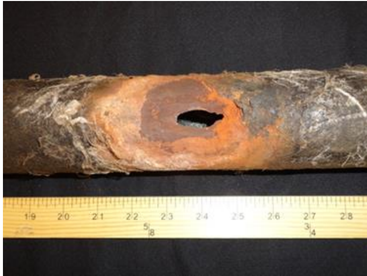
Figure 13: Photograph showing as-received perforated pipe sample.
