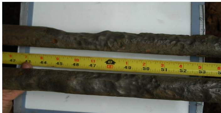
Figure 6: Dual round shafts of anchor AA. Maximum cross-sectional loss of 60% was measured on one of the two anchor shafts. Both shafts exhibited severe corrosion damage.
