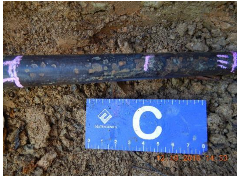
Figure 11: Photograph showing corroded anchor C.
