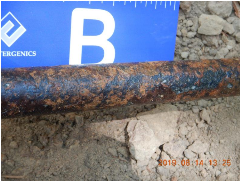
Figure 10: Photograph showing corroded anchor B.
