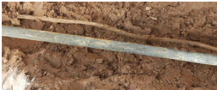
Figure 5: Single round shaft of anchor B. Galvanizing loss and minor surface corrosion below ground.
