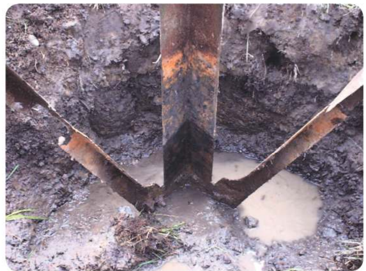
FIGURE 3 T&D towers are located in very corrosive and waterlogged soils with active bacteria present.
