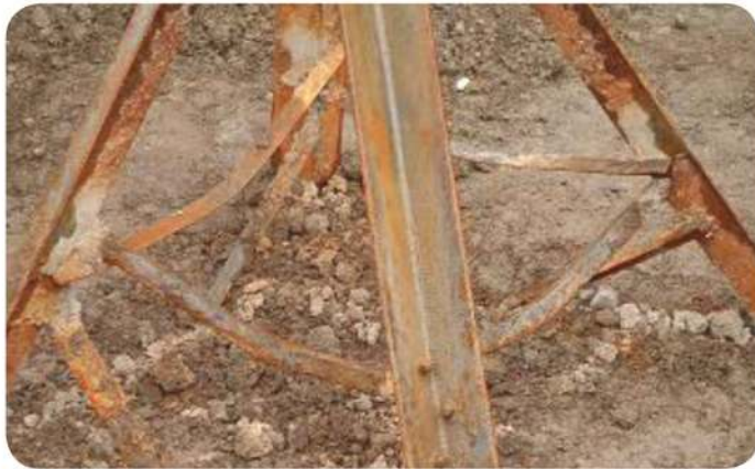
FIGURE 4 Heavy and corrosive backfills lead to accelerated corrosion of T&D towers.
