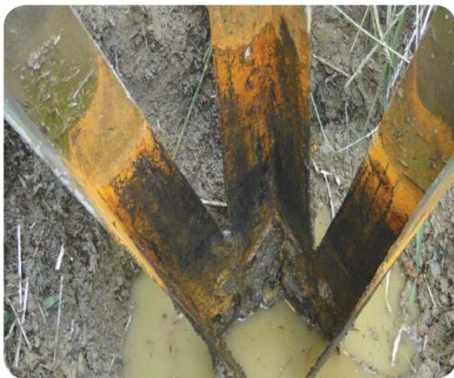
FIGURE 2 Transmission and distribution structures are exposed to all types of corrosion-inducing environments, including MIC, that require risk assessment.
