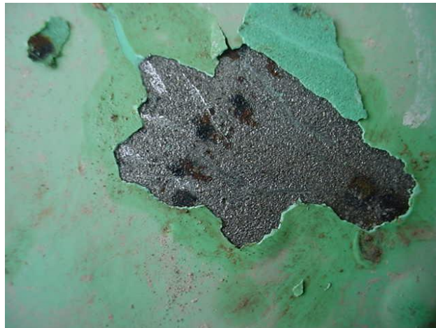
Figure 4: Disbondment of FBE coated pipe under cathodic protection.
