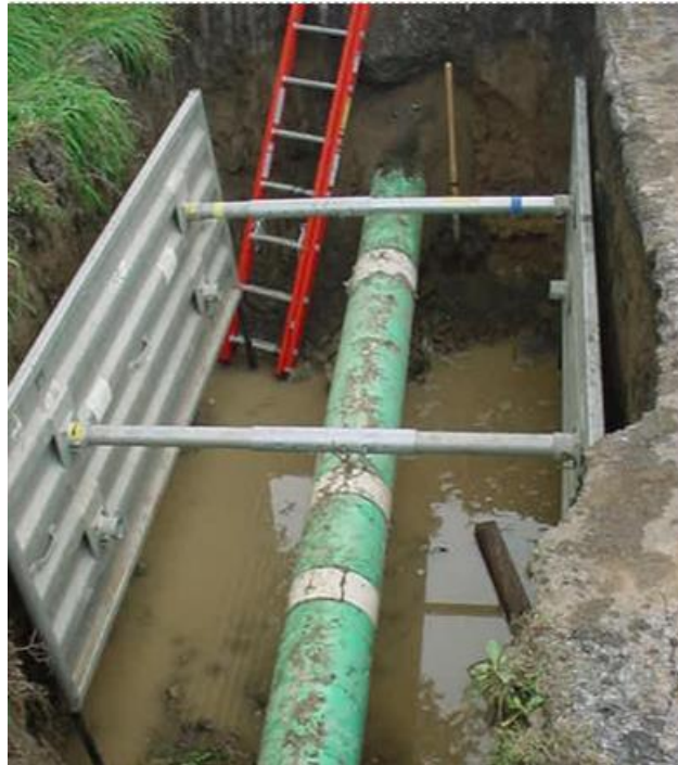
Figure 5: A fusion bonded epoxy (FBE) coated pipe and water table.
